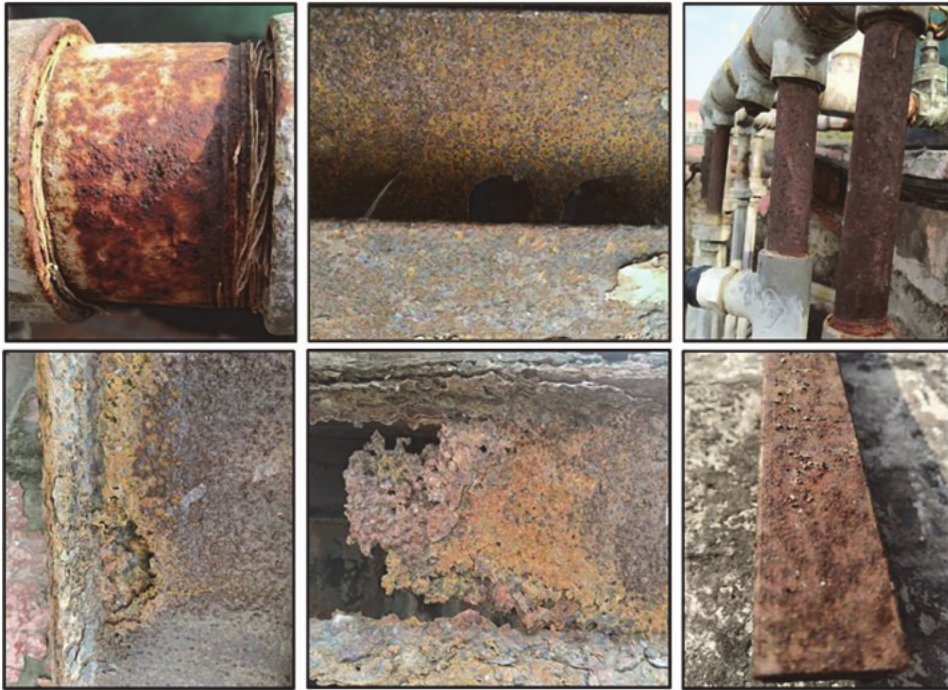
Figure 1. Effect of corrosion on different metallic structures.
