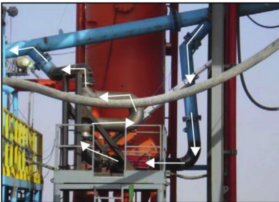
Figure 2. Coriolis installation on the bell nipple of a conventional drilling rig. N.B.: The arrows indicate the bypass and flow direction through the Coriolis from bottom to top [26].
