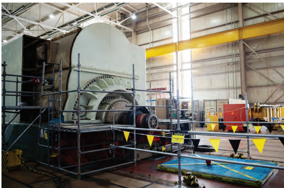
Part of the main generator inside the Crane Clean Energy Center.
