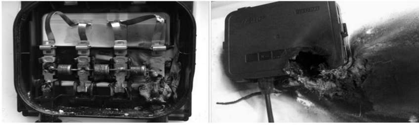
Figure 5.8 Burned junction boxes and bypass diodes [11].
