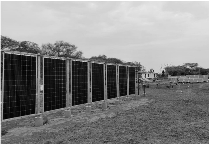
Figure 4.5 Vertically installed bifacial PV power plant at NISE.
