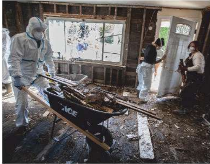
A gutted house in Swannanoa, N.C.
