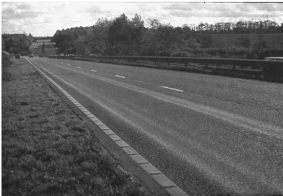
Figure 2 Serious rutting on a major highway.
