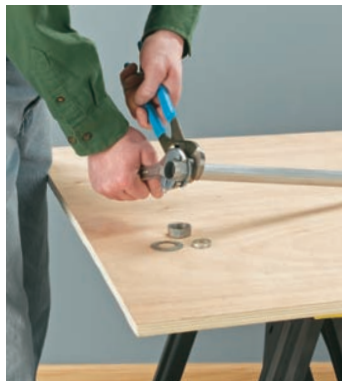
2. Insert the pipe into the compression coupling and tighten the fitting, using a channel-type pliers and adjustable wrench.
