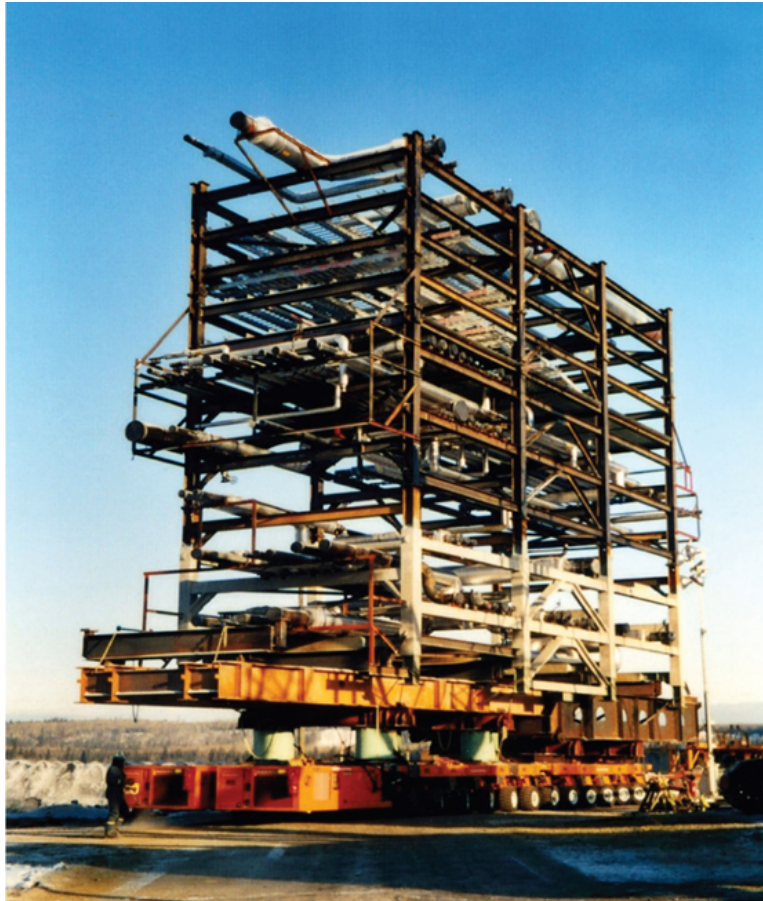
FIGURE 4.28 A Scheuerle multi-wheel transport platform, seen engaged in ground handling of a steel installation structure. The movement of such a load must be logistically planned, prior to the building/construction phase of the project.
