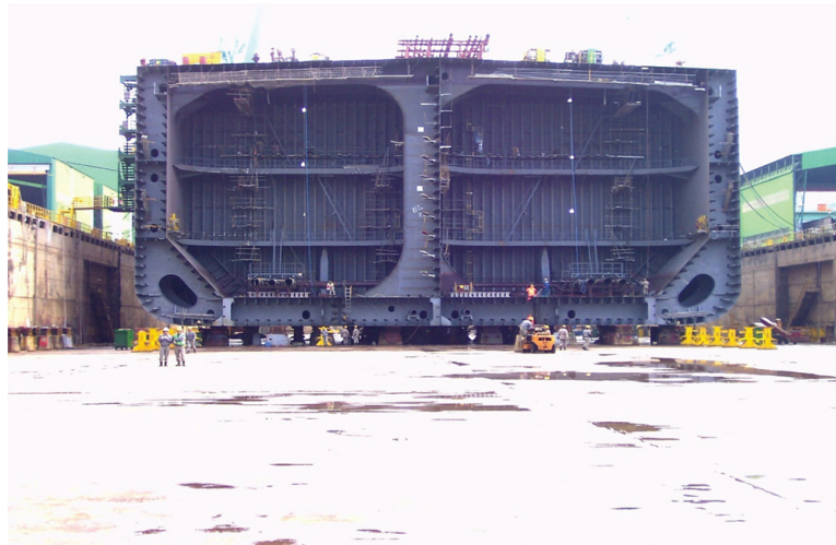
FIGURE 6.5 Athwartships cross-section of the modern double hull tanker seen at a late construction stage prior to assembly.
