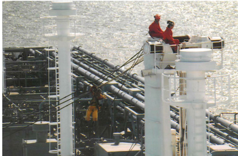
FIGURE 1.13 On-going maintenance of topping lifts, of derricks aboard a tanker vessel. Tankers generally have either derricks or cranes in an amidships position to lift pipe line connections on board close to the manifold. The derrick systems are usually supported by ‘Samson posts’ to accommodate tank venting and upper block securings.
