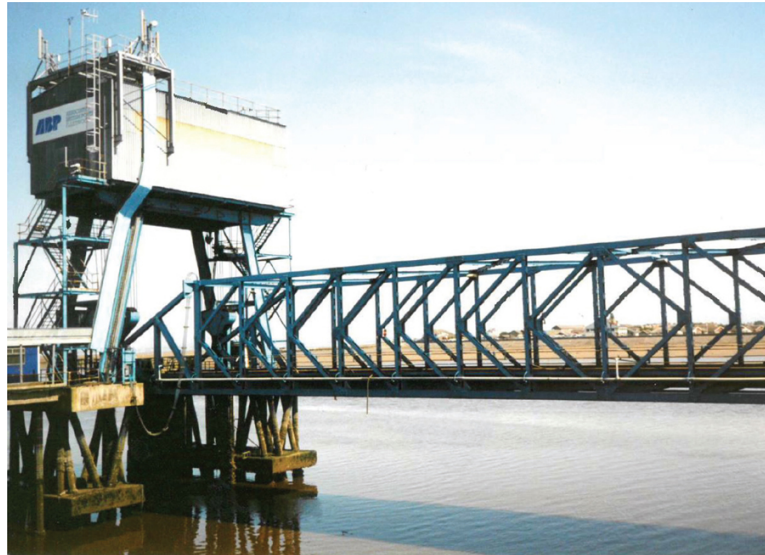
FIGURE 8.32 A typical mechanical link span machinery housing for hoisting and lowering the link span down to a position above the waterline. The stern ramp of the Ro-Ro ferry then lowers her stern ramp onto the links driveway to permit discharge of vehicles. The rise and fall of tide of 10.5 metres is countered by the adjustment of height to the link span to allow continuous operations no matter what state of tide.
