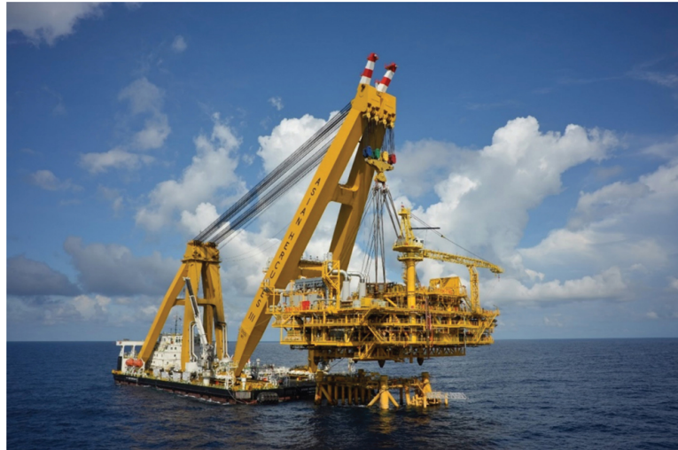
FIGURE 13.6 Asian Hercules II (IMO No. 8639297) a crane barge, floating sheerleg platform of the Asian Lift Pte Ltd, engages in a modular build up, to an offshore steel jacket of a developing offshore installation.
