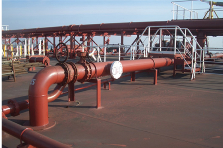
FIGURE 6.13 Deck pipeline example on the upper deck of an oil tanker.
