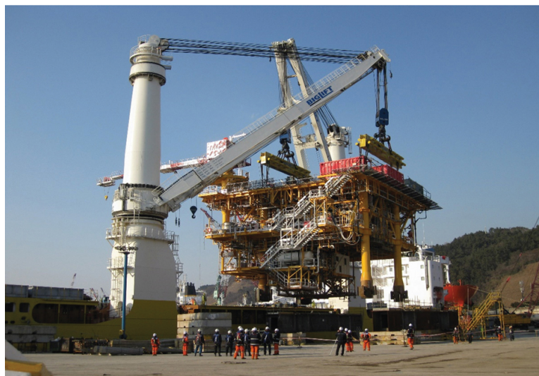
FIGURE 4.24 The ‘Happy Star’ (IMO No. 9661259) one of the Big Lift shipping company’s vessels engages in lifting a topside module by means of heavy duty lifting beams and a tandem lift by its two on board Huisman heavy lift cranes.
