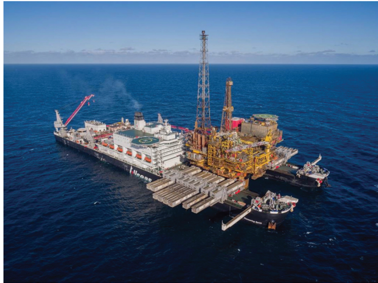
FIGURE 4.30 The world's currently largest ship Pioneering Spirit (IMO No. 9593505) has the equivalent deck space of six football pitches and has a lift capacity of 48,000 tons. In April 2017, the ship was engaged to lift the Brent Delta topside accommodation module, off the oil rig platform in the North Sea. The lift was 24,000 tons and was achieved in 12 hours by positioning the twin ballast hulls of the Pioneering Spirit under the rig and de-ballasting the ship to rise. (This lift holds the world's lifting record.)
