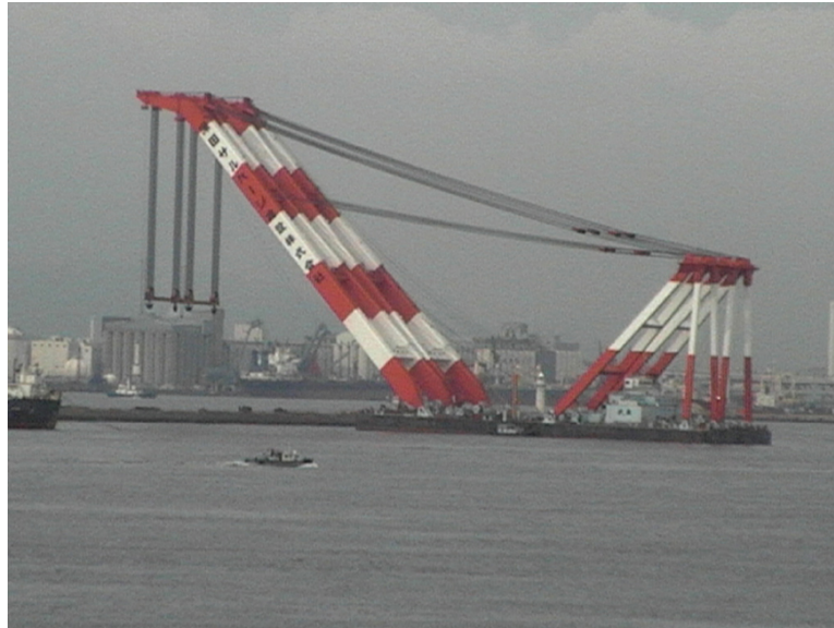
FIGURE 4.18 Heavy lift 'Sheer Leg' platform the 'Musashi' floating crane barge, seen off Kobe, Japan. This barge platform is towed to its working position. It has excessive ballast capacity for making extreme lifts up to 3,700 tonnes.
