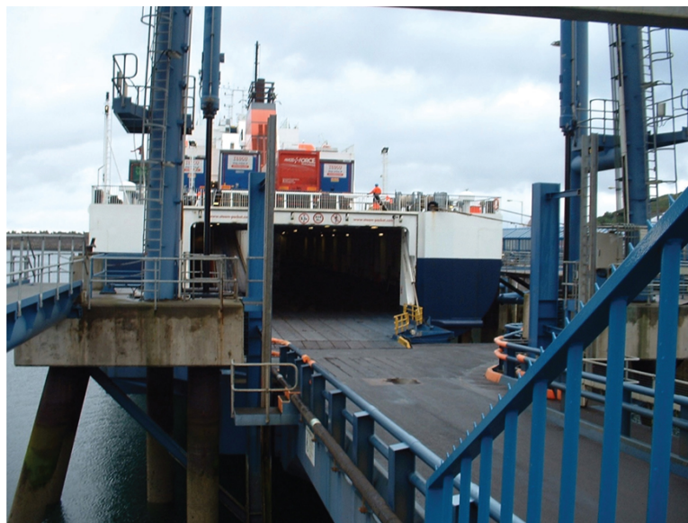
FIGURE 8.31 A typical road companionway adjustable link to a concrete structured dolphin at the port of Heysham, Cumbria. The height of the dolphin platform is built to accommodate the range of tide to allow acceptance of the vessels stern ramp. The ships stern door/ramp is then lowered for the angled flaps to lay flush to the companionway.
