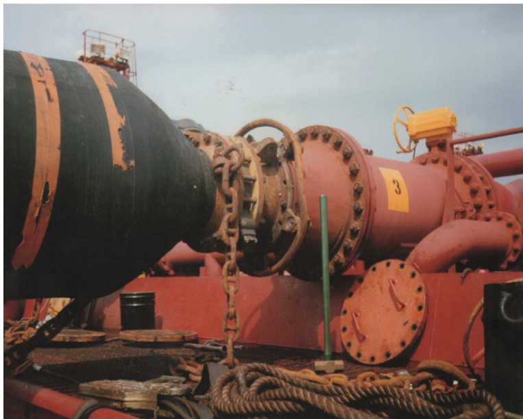
FIGURE 6.14 Manifold and pipeline connection. Typical 23-inch oil pipe connection.
