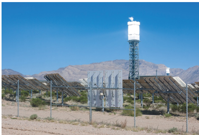
Figure 18.1 The Ivanpah tower and heliostat solar thermal project.
