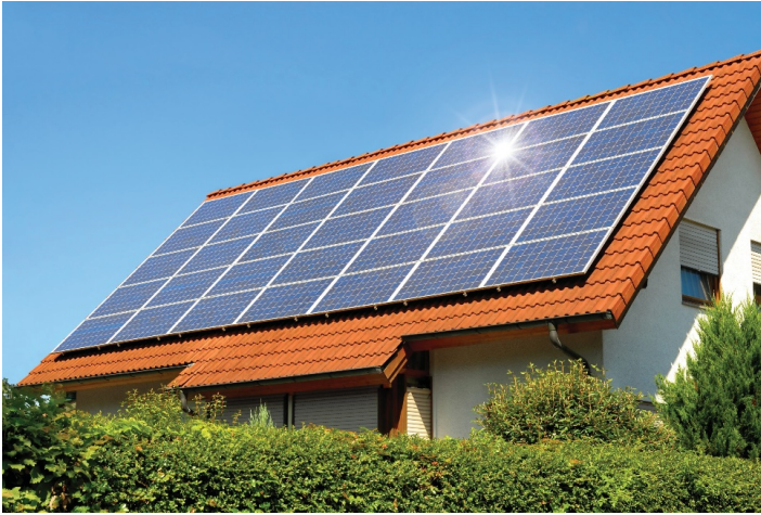
Figure 2.3 Ordinary crystalline silicon modules installed on a roof.
