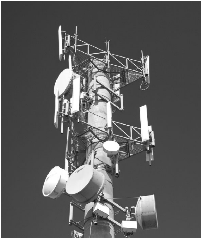
FIGURE 3.12 A microwave tower. The round antennas are microwave antennas and the straight antennas are cell phone antennas. Source: Matej, Pribelsky listock photo
