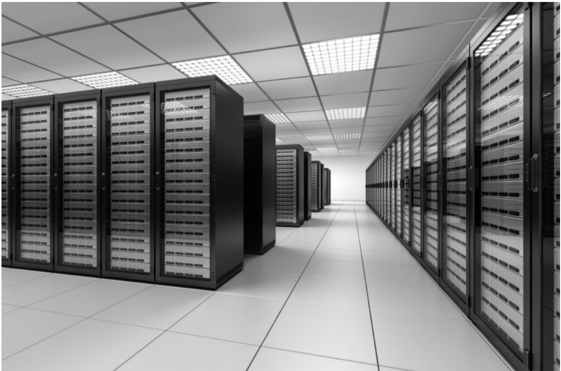
FIGURE 1.7 One server farm with more than 1000 servers
