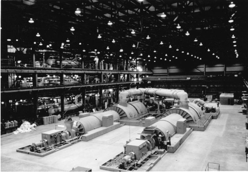
Figure 1.4 An installed 1300 MW cross-compound turbine generator.
