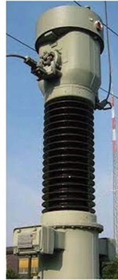
(b)- Current transformer
