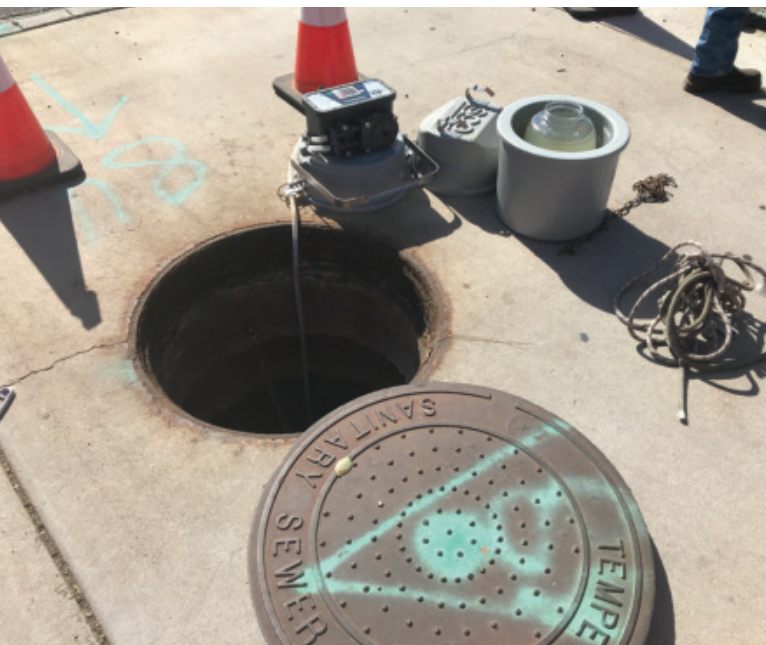
A small automated machine perches at the edge of a maintenance hole, ready to retrieve wastewater samples (like the one in the gray container) from the Tempe, Ariz., sewage system.
