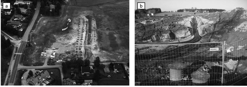
FIGURE 4.17 (a) BTES at Ahus under construction in the summer of 2007; (b) boreholes to manifold pipelines at Ahus (Midttømme et al. , 2009).
