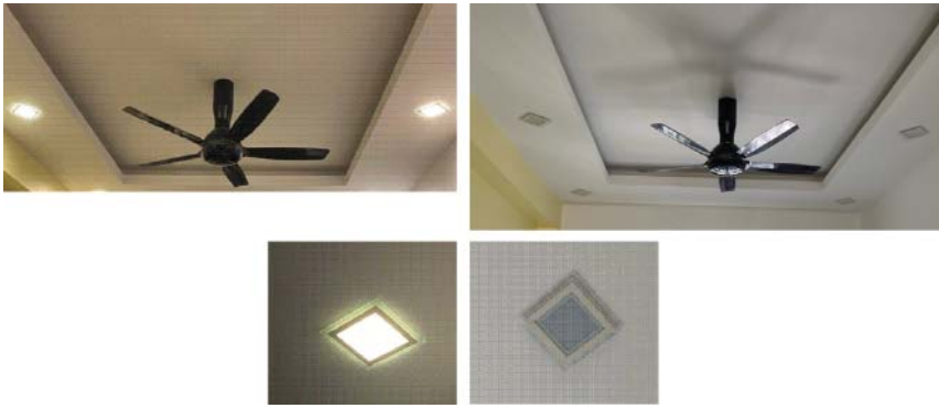
Figure 6.8 Retrofit square-shaped LED downlight in the living room.
