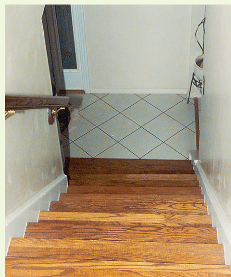
STEP 2k Handrails installed along stairways provide security for patients with visual, balance, and coordination problems.
