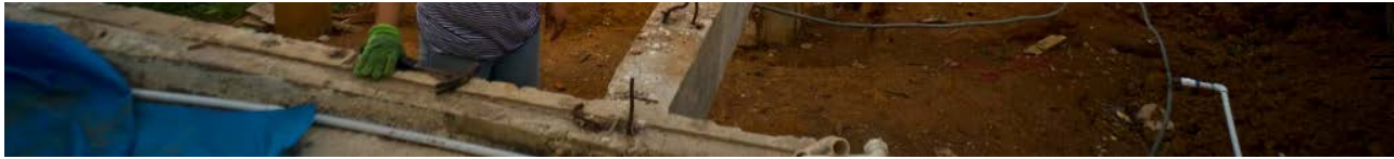
Alma Morales Rosario poses for a portrait between the beams of her home being rebuilt after it was destroyed by Hurricane Maria one year ago in the San Lorenzo neighborhood of Morovis, Puerto Rico, on Sept. 8, 2018. Photo: Ramon Espinoza/AP
