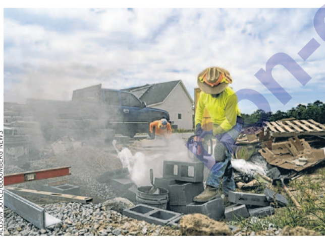
A new subdivision under construction in Raleigh, N.C., another city where housing has become much less affordable
