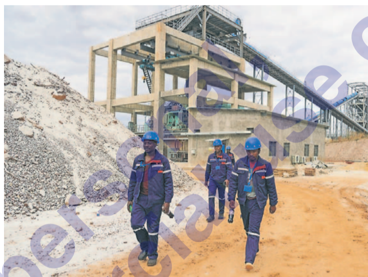
Components of renewable energy technology are concentrated among a few top producers; a lithium mine and processing plant in Zimbabwe.
