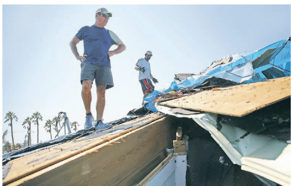
Damage from Hurricane Irma in Sugarloaf Key, Fla., in September 2017.
