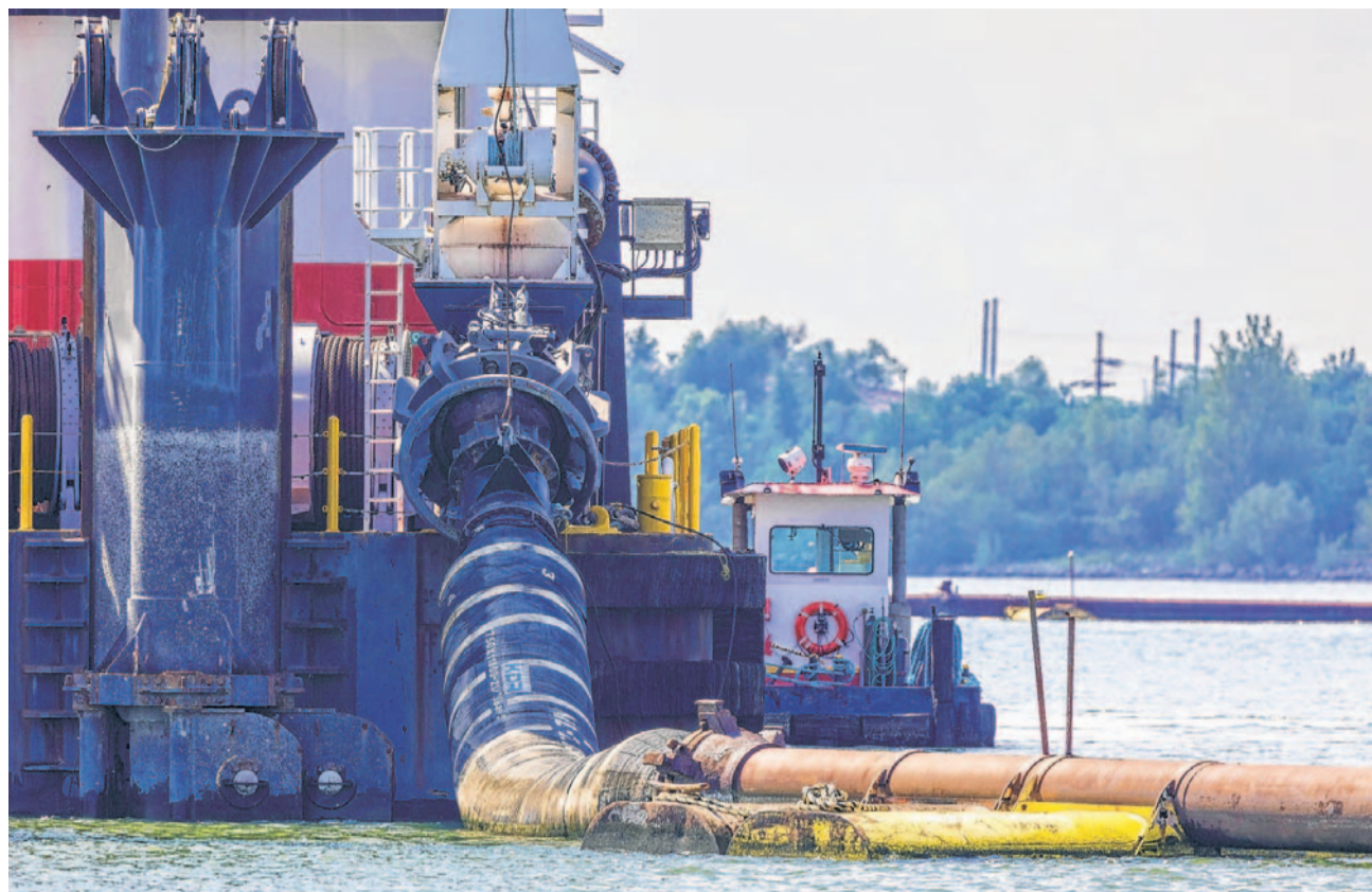
A pipe pulled and transported sediment from the Mississippi River south of New Orleans last week.
