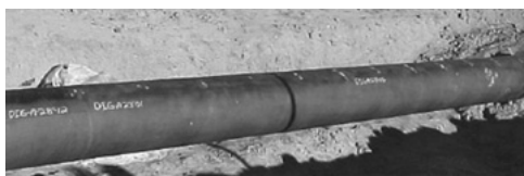
FIGURE 6. Carbon steel, 0.75 m (30 in.) outside diameter, gas transmission pipeline.
