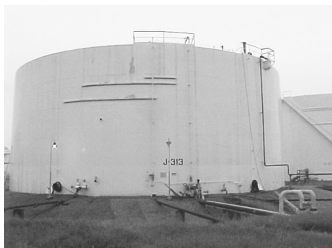
FIGURE 8. Aboveground storage tank for petroleum products.
