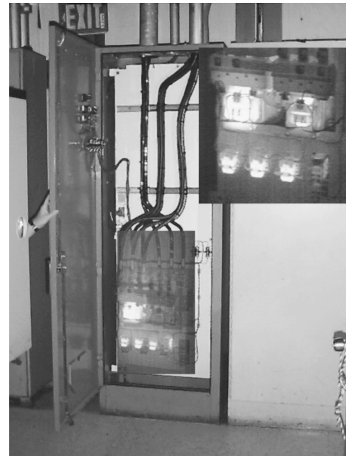
FIGURE 11. Infrared thermography of automatic transfer switches of emergency diesel generator. Hot spots appear bright in thermogram (inset).
