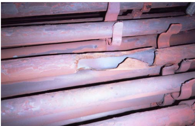
FIGURE 9. Boiler tube failure from creep in reheater tubes. Inside diameter oxide measurements taken using high frequency ultrasonic tests are used to calculate remaining creep life.
