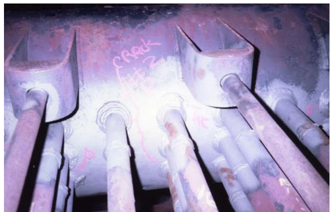
FIGURE 10. Inspection of a header in fossil plant. Ultrasonic testing can be used to detect ligament cracking between tubes if there is enough spacing between tubes for transducer placement.
