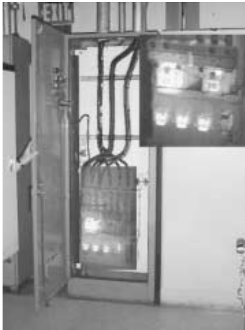
FIGURE 9. Infrared thermography of automatic transfer switches of emergency diesel generator. Hot spots appear bright in thermogram.
