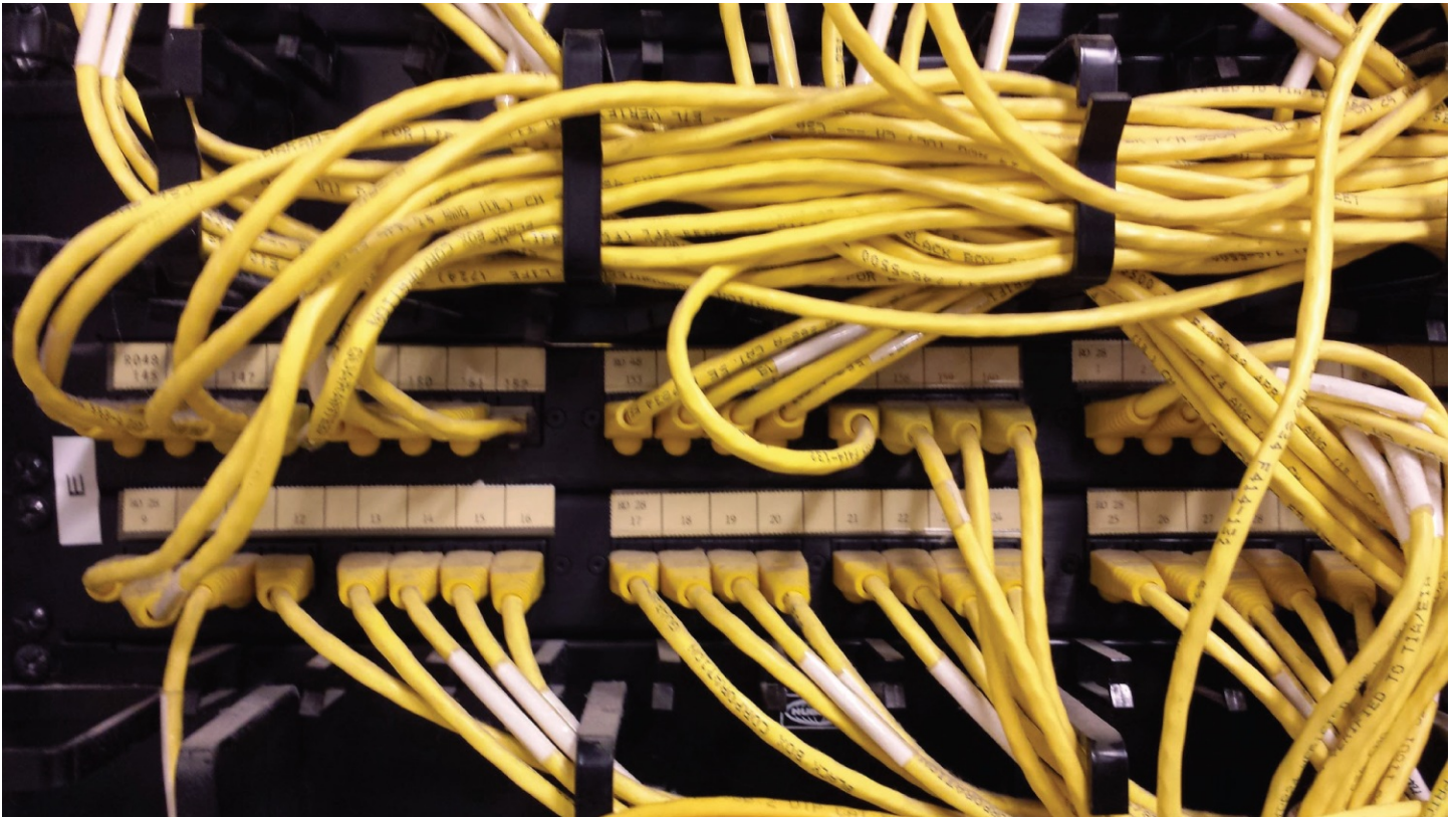
FIGURE 1.54 Cable management example
