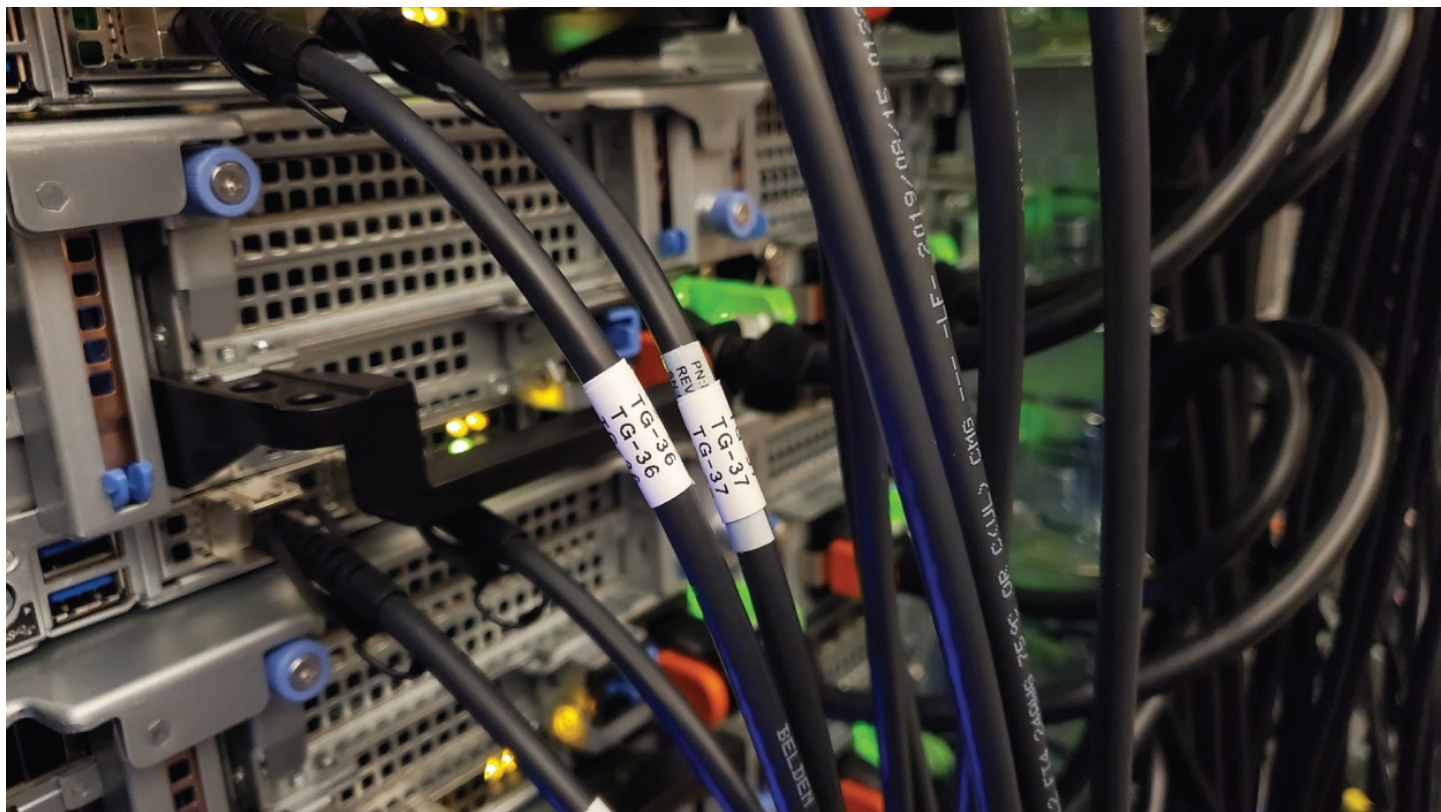
FIGURE 3.19 Network cable label wrap
