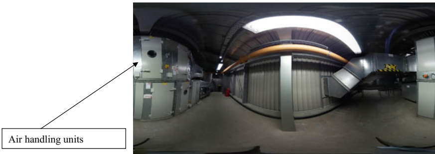
Photo 4 A plant room containing air handling units in room 10
