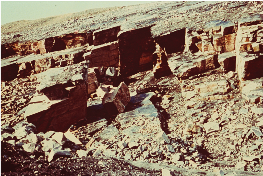
Figure 2.1 Image of rock slope in sandstone containing persistent bedding dipping at 30°–35°, with blocks sliding on bedding.
