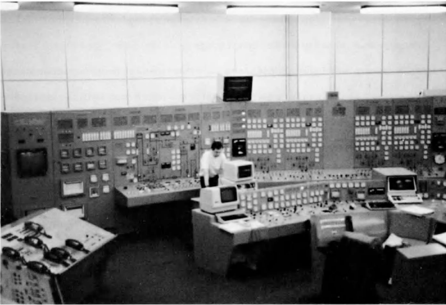
Figure 5.3 : Simulator Control Room
