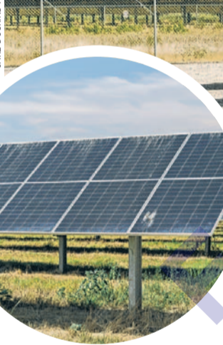
Battery storage at an Enel solar facility in Texas this month. In the state, which logged 10 demand records this summer, batteries helped avoid rolling blackouts one recent evening.
