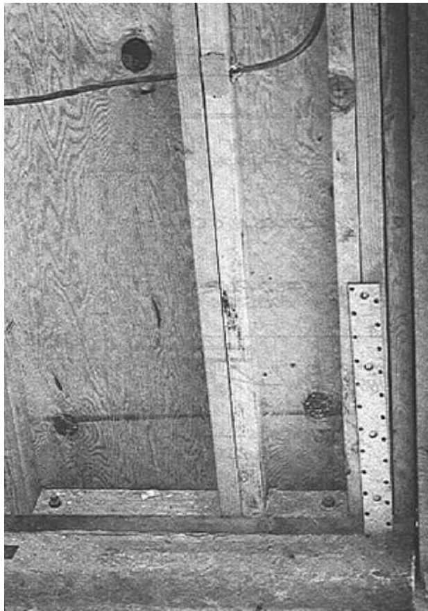
Figure 13-5. Hold-down straps are used in addition to anchor bolts in an earthquake zone.
