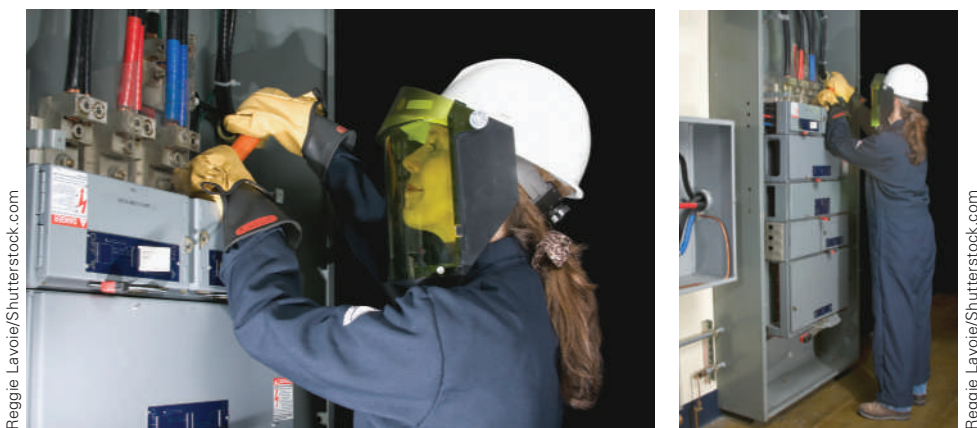
FIGURE 11-6 An example of the personal protective equipment required during the majority of industrial electrical tasks.
