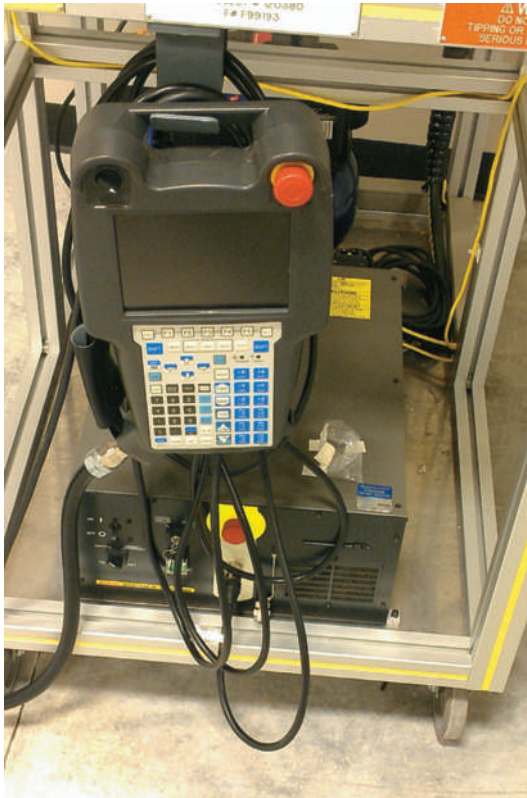
FIGURE 1-2 The teach pendant for the FANUC trainer. Note the big red E-stop on the upper-right corner of the teach pendant as well as the E-stop on the controller directly below the teach pendant.
