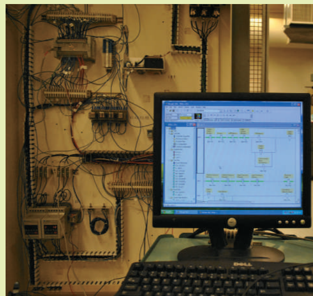
FIGURE 9-16 The control cabinet as well as some of the PLC program driving the system.
