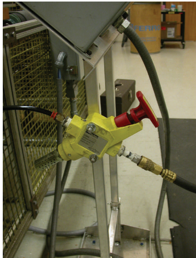
FIGURE 1-15 This disconnect for an air system would require attention during the LOTO process.
