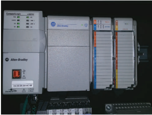
FIGURE 10-5 An Allen-Bradley CompactLogix controller. Notice the LED section on the upper-left side. While the specific location and lights may differ from brand to brand, they all should have some means to give technicians information about the system at a glance.
