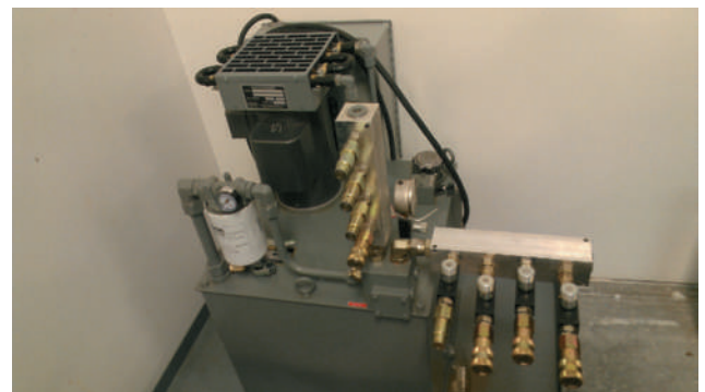
FIGURE 11-4 This stand-alone power unit is used in various fluid power labs. The white canister on the left is the filter. The cooling unit is located on top of the pump motor. Both the filter and the cooling unit require yearly maintenance.
