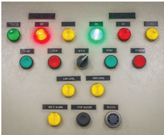
FIGURE 10-10 A simple control station with several indicator lights, a few pushbuttons, and a selector switch in the middle.
