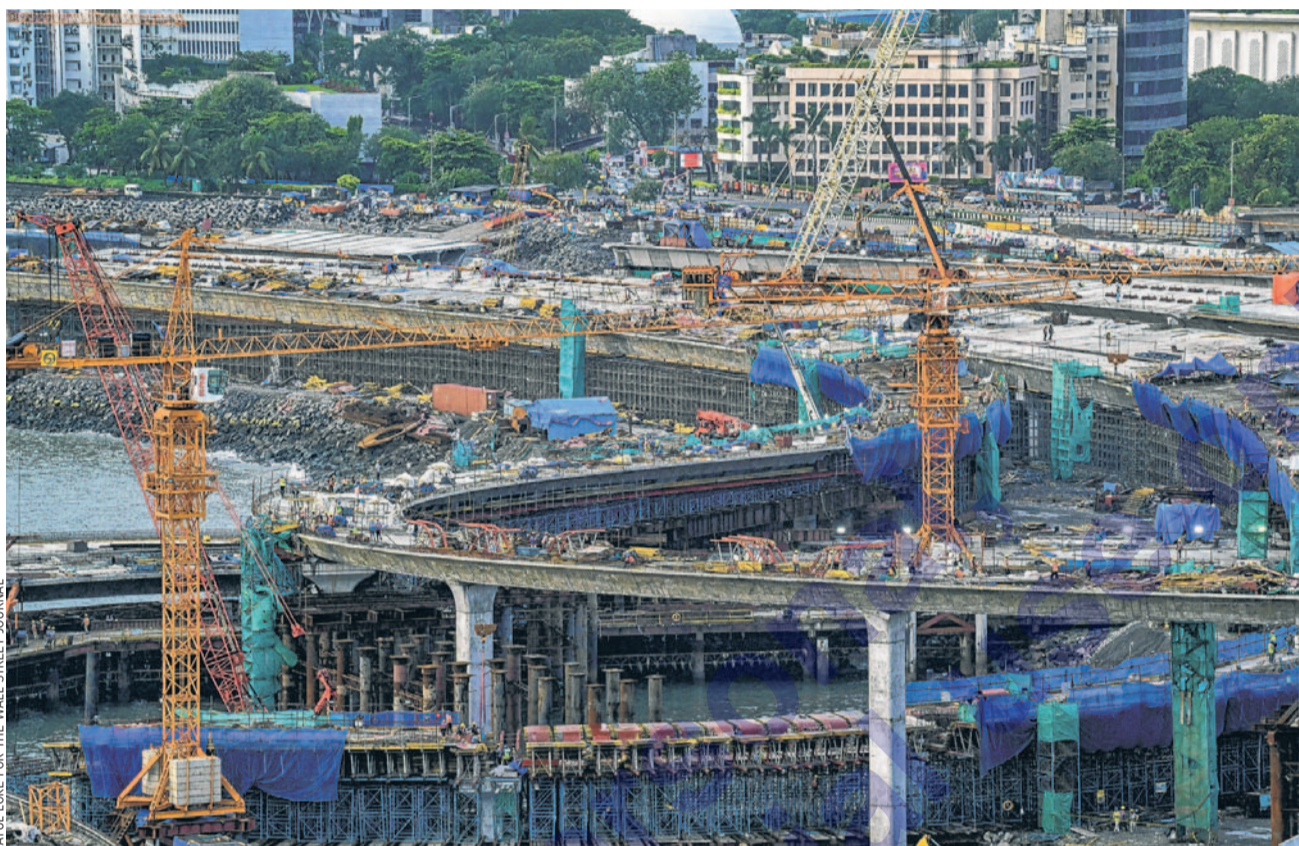
A coastal-road construction site in Mumbai. Hundreds of miles of new roads are being added every month in India.
