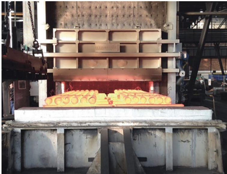
Fig. 6.14 Bogie hearth furnace for semi-finished rolled products. (Foto: Kopsch, St., BGH Edelstahl Freital GmbH)
