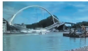
(o) Nan Fang'ao bridge in Taiwan, collapsed in 2019, corrosion [27]
