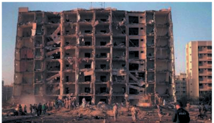
(g) Khobar tower in Saudi Arabia, collapsed in 1996, bombing [20]
