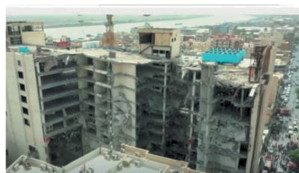
(q) Metropolis building in Iran, collapsed in 2022, poor construction and overloading [29,30]
