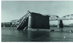
(b) Silver bridge in Ohio, collapsed in 1967, corrosion [15]
