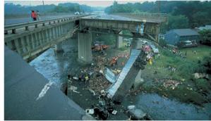
(e) Mianus River bridge in Greenwich, collapsed in 1983, corrosion and poor maintenance [18]
