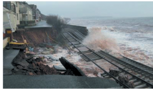
(k) Sea wall at Dawlish, UK, collapsed in 2014, storm [22]
