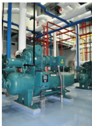
Industrial ammonia refrigeration system.
