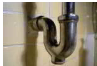
A sink drain can become clogged with saturated fats.
