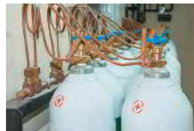
Cylinders of oxygen gas are placed in a hospital storage room.
