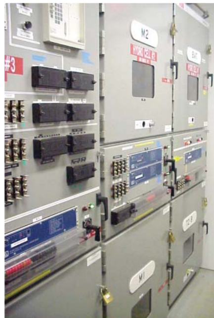
Figure 11.22 Protection devices on arc-proof metal-clad cell doors.
