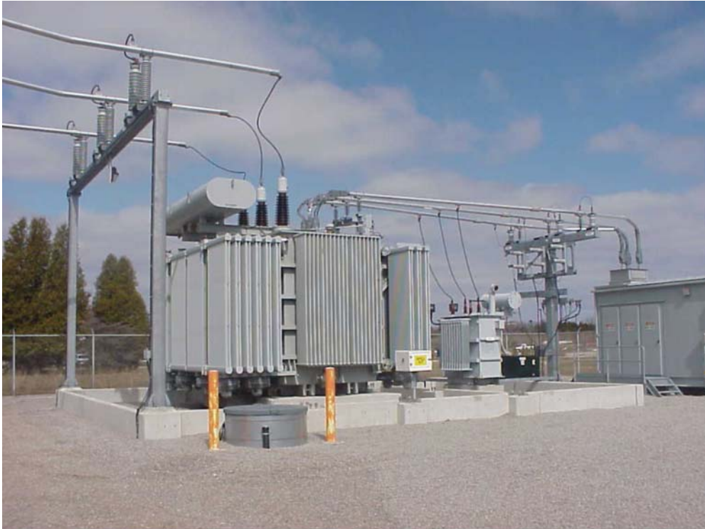
Figure 8.1 33 MVA 115–13.8 kV Power Transformer.
