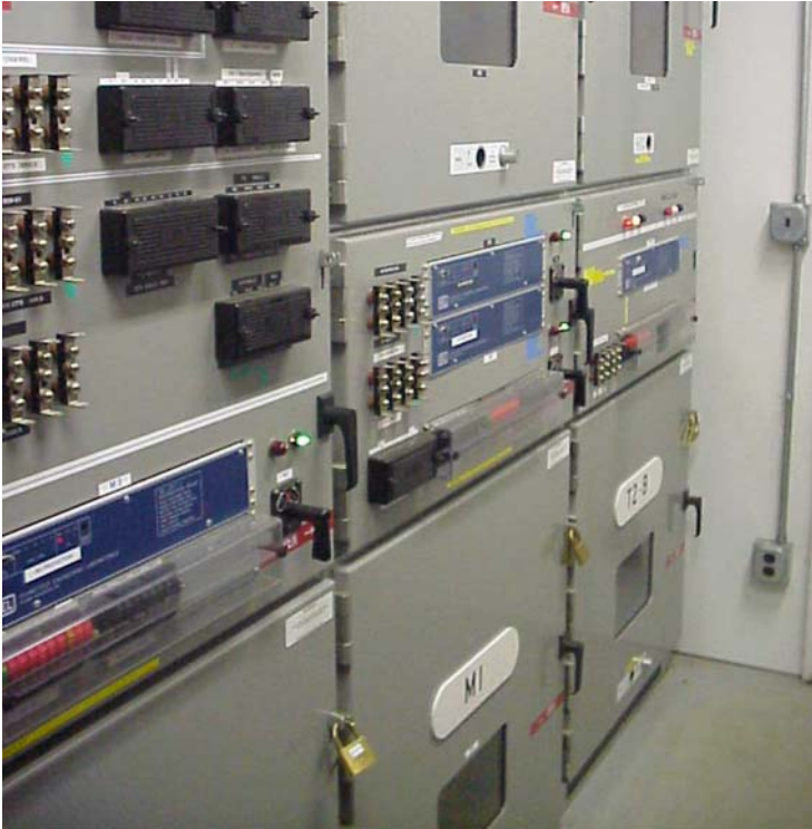
Figure 9.35 Bus and feeder protections mounted on metal-clad switchgear.
