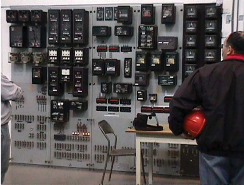
Figure 2.6 A set of legacy protection panels on several racks for a line protection system.
