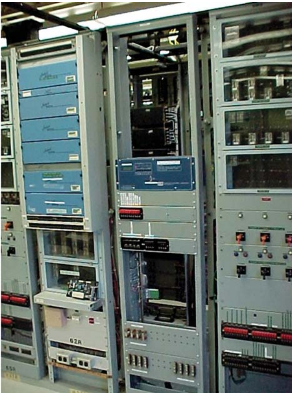
Figure 5.7 Digital relay interfacing with telecommunication equipment.
