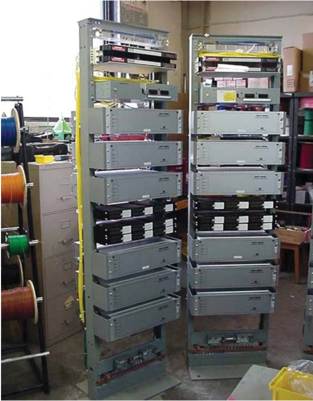
Figure 2.9 Digital telecommunication equipment used for line protections.
