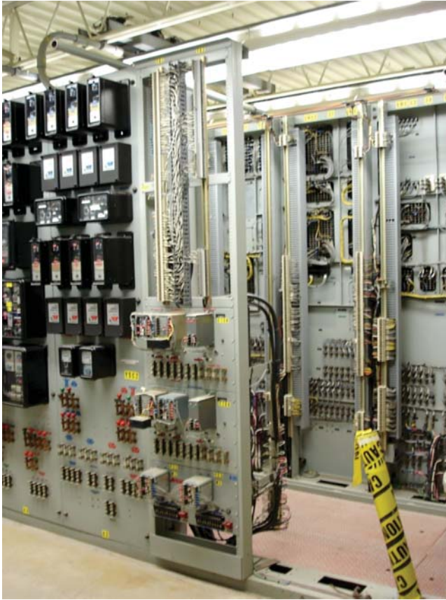
Figure 2.10 An illustration of relays, panels, terminations, wiring, and isolation switches.
