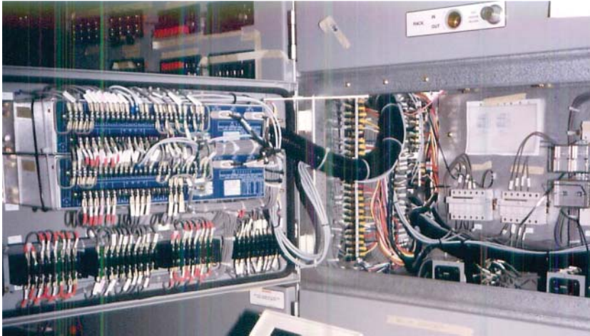
Figure 11.23 Backside view of a metal-clad instrument compartment.
