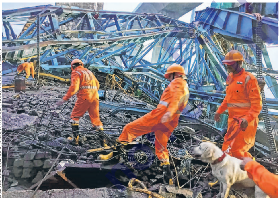
SEARCH FOR SURVIVORS: Rescue workers search the debris after a crane collapsed in Thane, India, on Tuesday, killing at least 16 construction workers.
