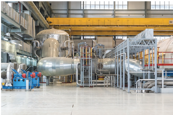
FIGURE 13.18 The turbine hall of a nuclear generating station. The large silver tanks are separators that remove water from the steam after it has left the high-pressure turbine and before it is recycled back into the low-pressure turbines.
