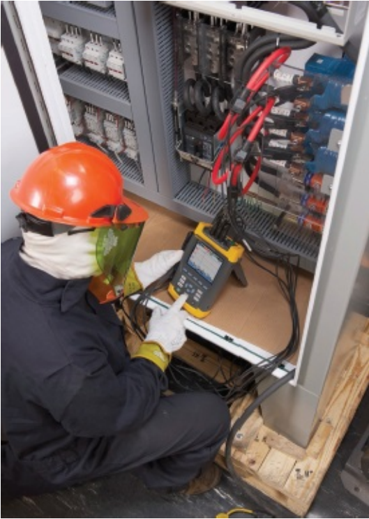
Figure 10-36 Taking measurements on a VFD.
