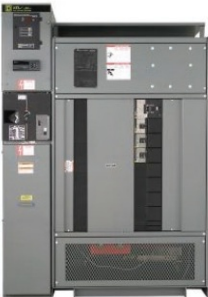
Figure 3-4 Factory assembled unit substation.
