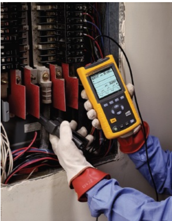
Figure 5-44 Power quality analyzer.
