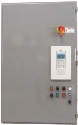
Figure 10-23 Typical VFD package.
