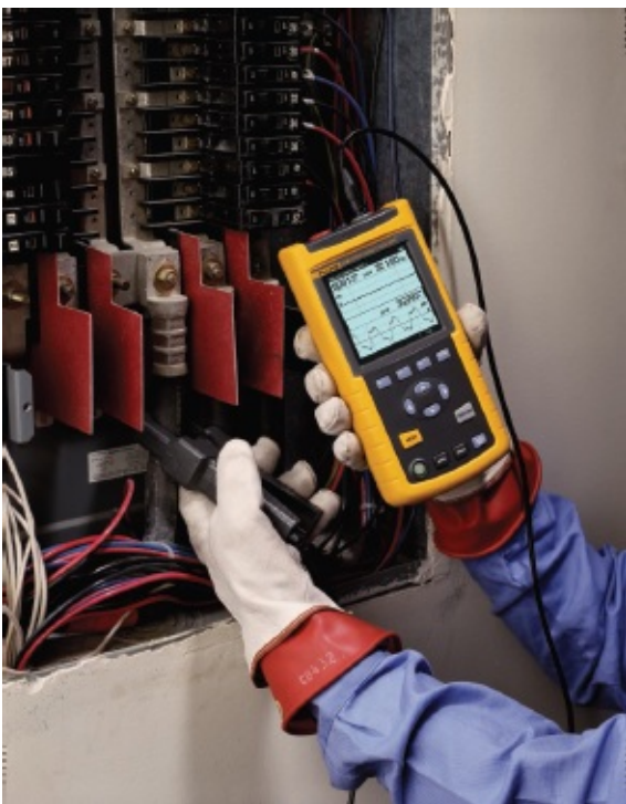
Figure 5-44 Power quality analyzer.
