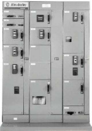
Figure 3-16 Typical motor control center.
