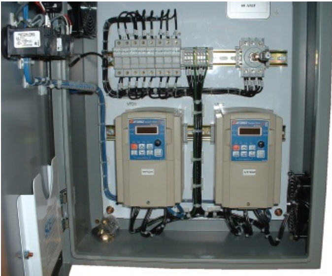
Figure 10-17 VFD mounted within an enclosure.
