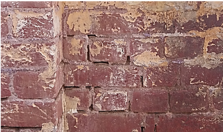
FIGURE 7.3 Wall of heritage structure facing degradation of binding material.
