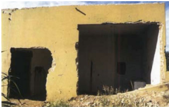
Fig. 2 The bunker remains after it was vandalised. Reproduced with permission from International Atomic Energy Agency, The Radiological Accident in Goiânia, IAEA, Vienna (1988)
