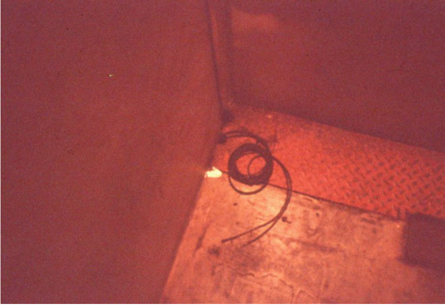
Fig. 4 Cables that should have been connected to a Geiger counter
