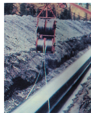
Figure 14.6 Zinc wire is attached to this underground pipe at intervals of 500 to 1000 ft. The zinc loses electrons more easily than the iron and is, therefore, oxidized instead of the iron.
