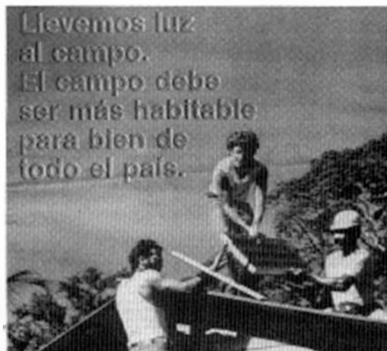
Local Dominican solar technicians installing a module. The Spanish reads: "We bring light to the countryside. Rural areas ought to be made more habitable for the good of all the country."
