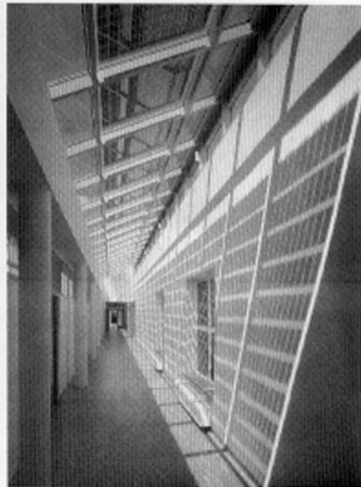
These solar modules also shade the interior from the excessive heat of the summer sun.
