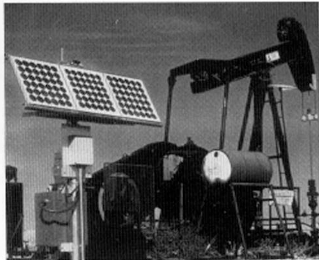
Solar electricity protects this wellhead in Kansas from underground corrosion.
