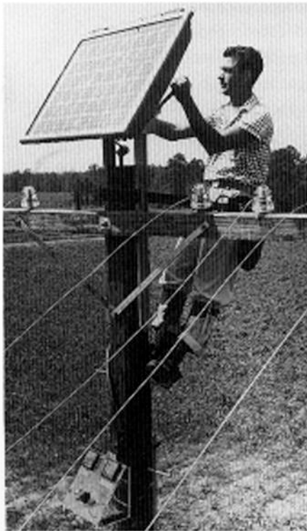
A hneeman installing a Bell solar array to power a rural telephone line in Americus, Georgia.
