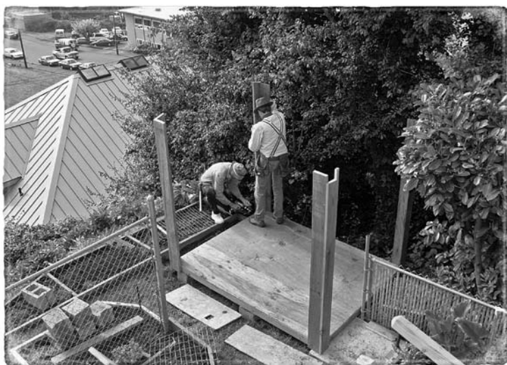
Single-wall construction starts by screwing boards to the outside of the floor frame.
