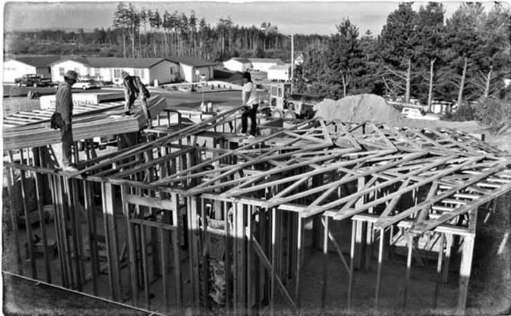
Using trusses to build roofs simplifies what used to be a more challenging job.
