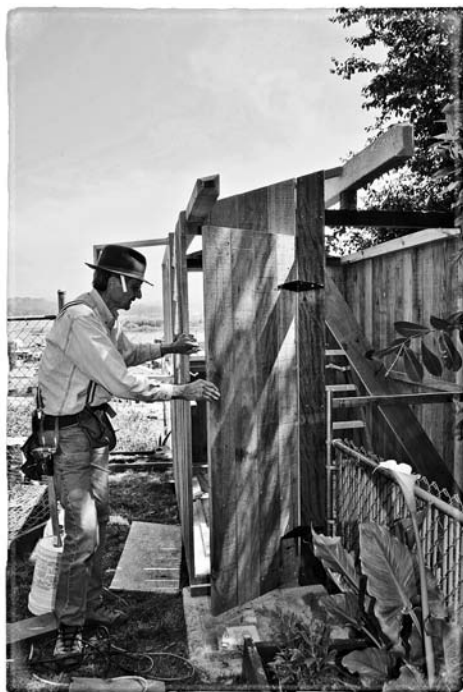
A different type of prehung door, made from the same material as the greenhouse and hung in place with a couple of strap hinges.
