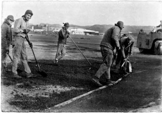
We were laying asphalt for a taxi strip at an American base in Newfoundland (I am second from left). You can just make out a Quonset hut in the background.
