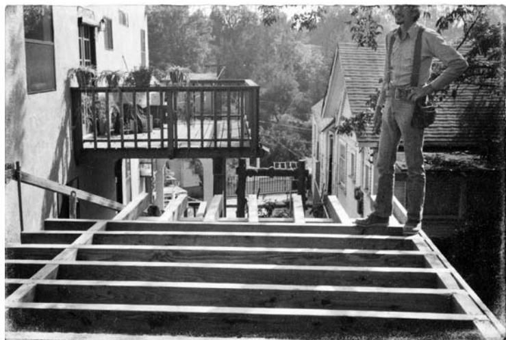
With the foundation gone, I excavated and built a small room under the garage. The joists became the deck of this garage and the ceiling of my writing room.
