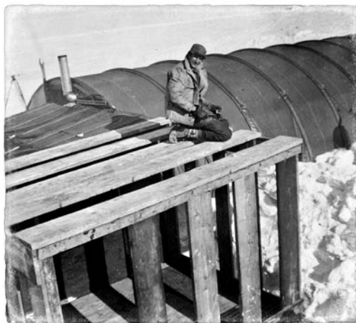
We built a structure out of 2×12s for a shower room and toilet.
