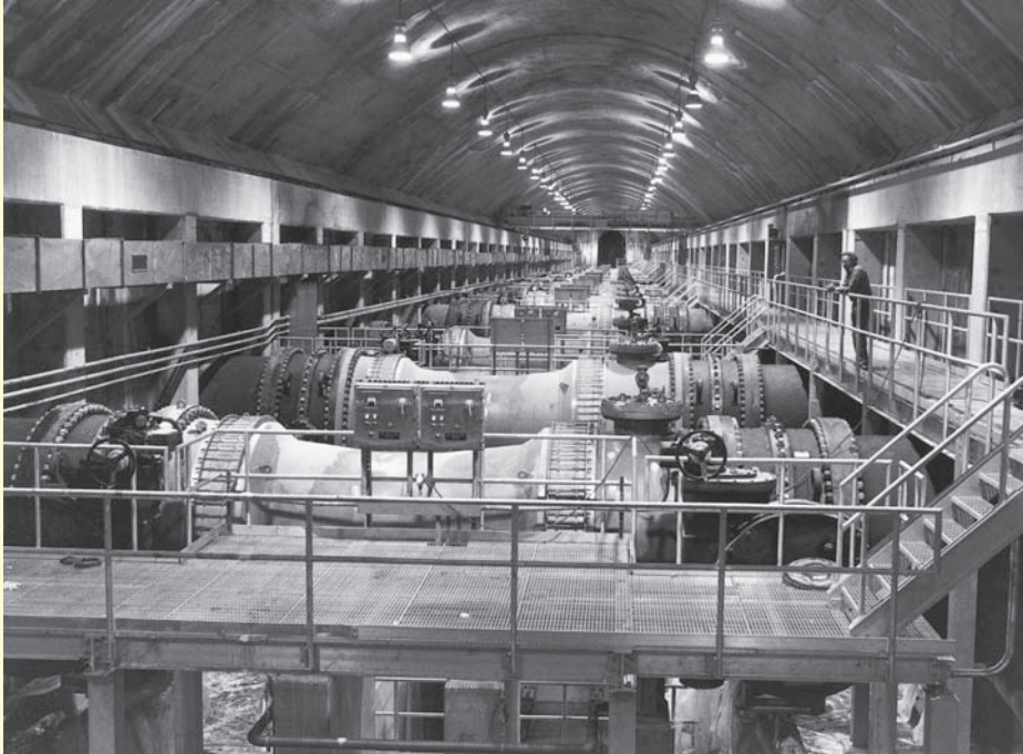
The valve chamber in Van Cortlandt Park was completed in the early 1990s. Photo courtesy of New York City Department of Environmental Protection
