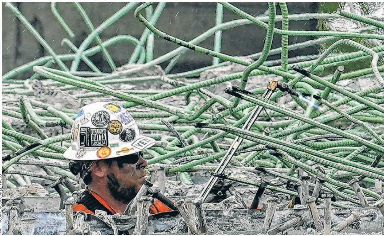
TRAFFIC SNARL: Pennsylvania officials said Wednesday that 2,000 tons of lightweight glass nuggets will be used to help rebuild and reopen a collapsed section of Interstate 95 in Philadelphia. Above, a worker cuts mangled reinforcing bars there.
