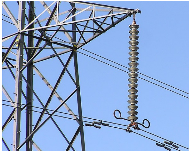
FIG. 3.22 Suspension insulator. Source: Wikipedia.
