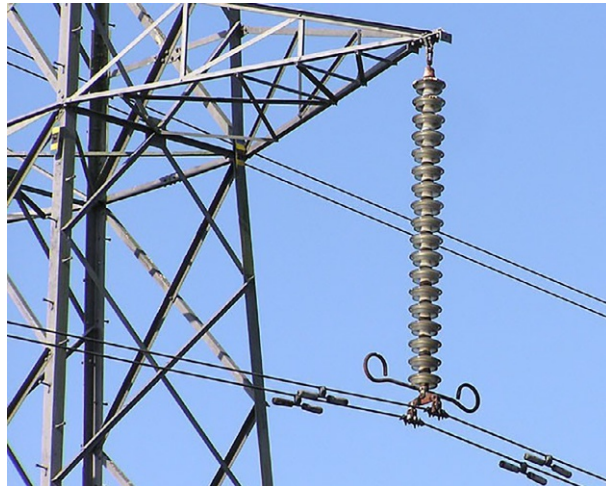
FIG. 3.22 Suspension insulator. Source: Wikipedia.
