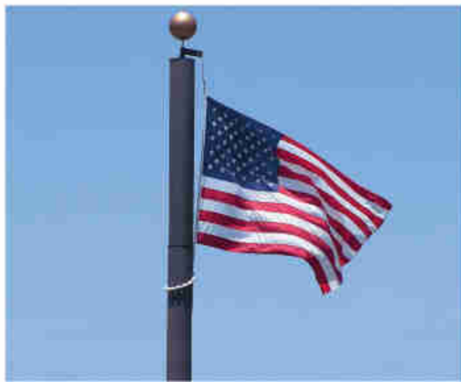
The flag's real. The pole's a cellular tower.
