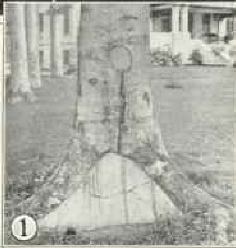
1 A crude cement patch—ineffective and injurious.
